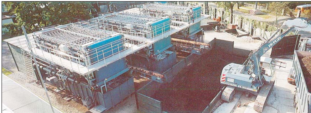
Dehydrating plant in Falkensee combined with a filtrate water purification plant with an output of 300 m 3 /h
